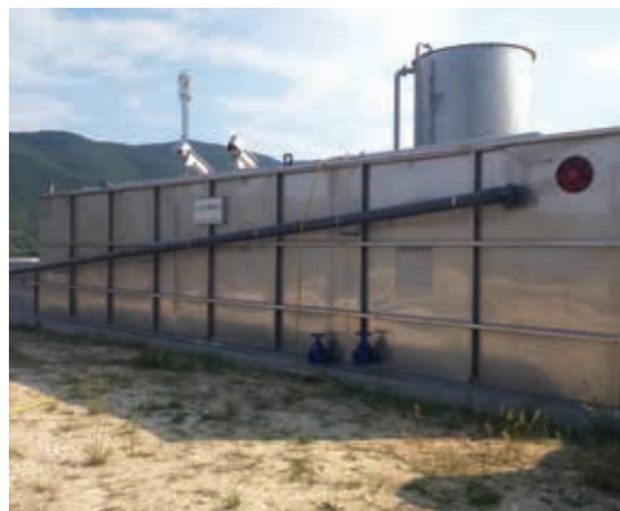
Compact MBBR Unit
