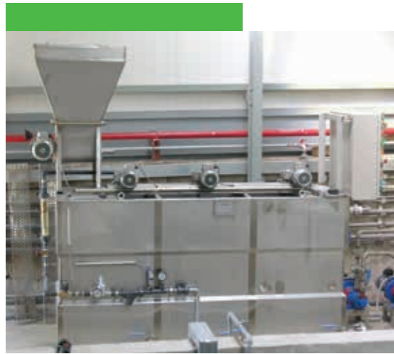
Polyelectrolyte Preparation Unit
